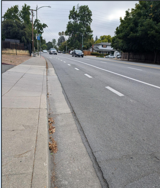
Bike lane markings faded
